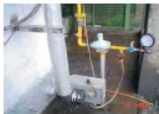
Photograph of LPG connection
