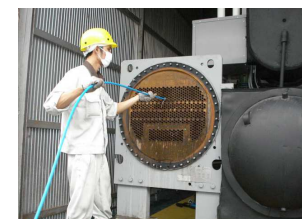
Fig 2.7 Cleaning chiller machine on scheduling
