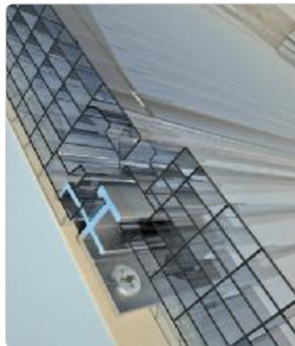
INSERTION OF PLATE Insertion of aluminium plates for anchorage to existing structures.
