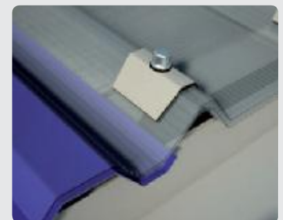
ANCHORAGE OF ROOFING This is done by drilling and inserting a screw with Vipla washer and cap.
